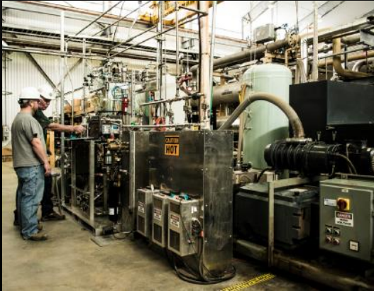
Extraction of UAr at Colorado. Crude argon gas mixture (Ar, N 2 and He)
